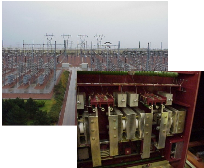
IFA 2000 station de redressement HVDC France-Angleterre (Thyristors)
